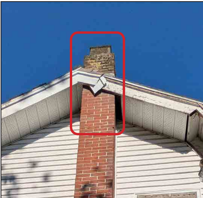
Fig. 13a: View of the side elevation brick chimney, 2025, showing its fair condition at the top and its largely good condition along the side. (Source: Cummer)
